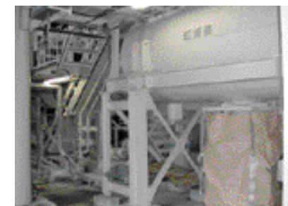
Machine for drying calcium fluoride sludge
