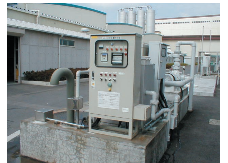
pH neutralizer installed by Toyo Takasago Dry Battery.
