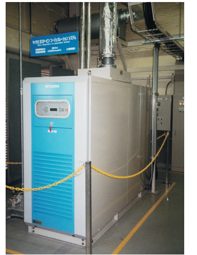
Micro-gas turbine co-generation system installed at OSRAM-MELCO Co., Ltd.
