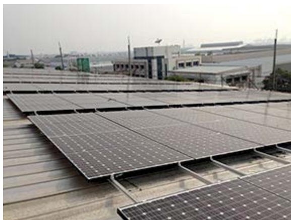
Photovoltaic system introduced at Siam Compressor Industry Co., Ltd.
