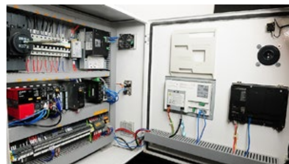
Single-interface control of the entire building through BMS.
