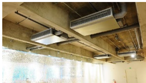
Precision control of heating, ventilation and air-conditioning.
