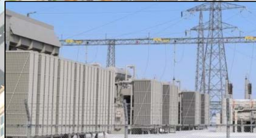
Power Distribution Facilities
